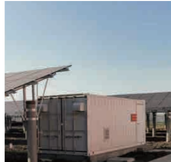
Microgrid Project Nanjing, China
