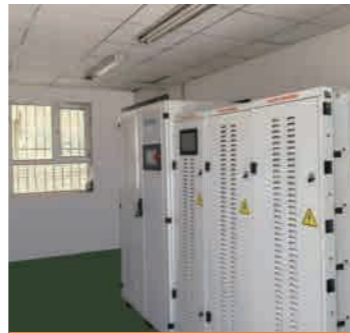
Microgrid Project in Torugart Port, China
