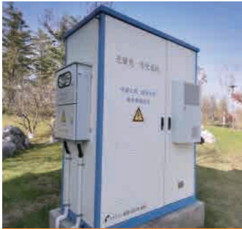
PV-ESS-EV Project in Henan, China
