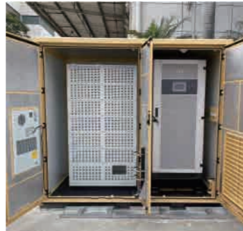
Microgrid Project in Sierra Leone, Africa
