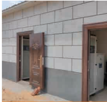
Microgrid Project in Yulin Coal Mine Area, China
