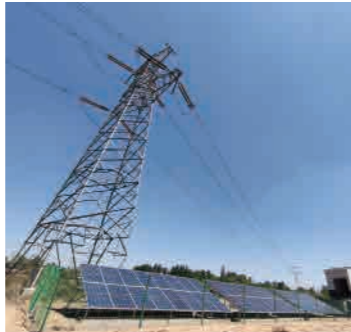
Microgrid Project in XinJiang, China
