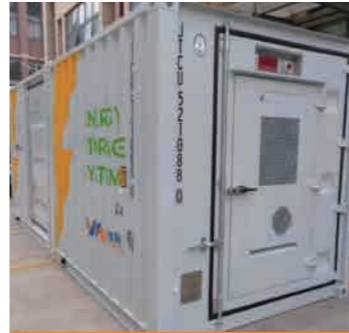
Microgrid Project in Pakistan
